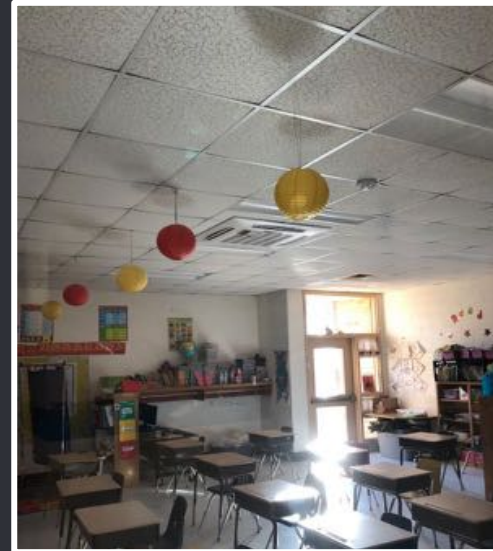
Jefferson Parkway LED Lighting
