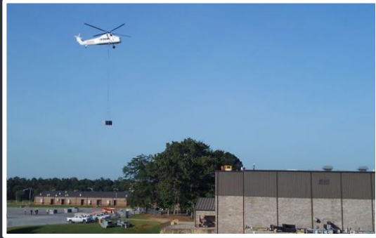
High School Gym HVAC Delivery
