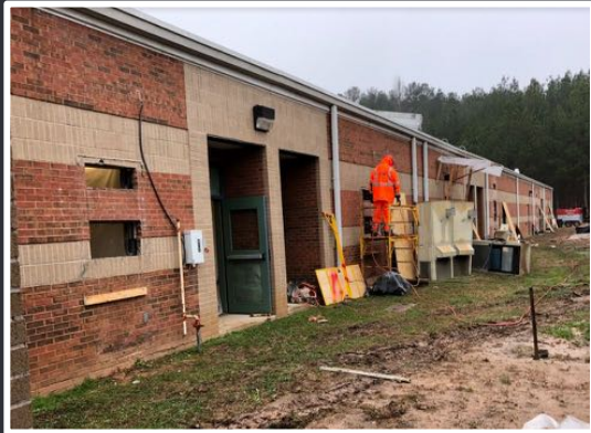
Newnan Crossing HVAC Update
